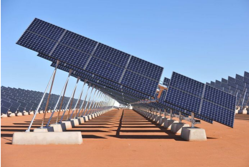
PHOTO: The Alice Springs power system was unable to cope with a minor cloud over the Uterne solar farm. (Supplied: Epuron)
